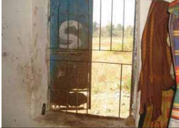
Broken windows and other poor infrastructure of hostels a common sight
