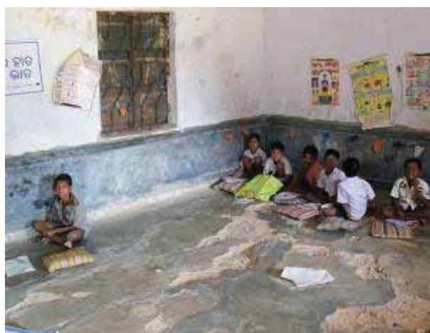
Chipped and dusty classroom floor
