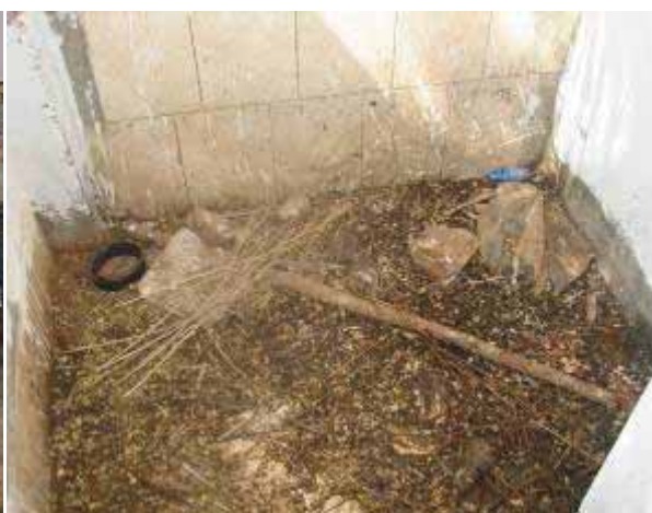
Dirty or non-functional toilets a common sight
