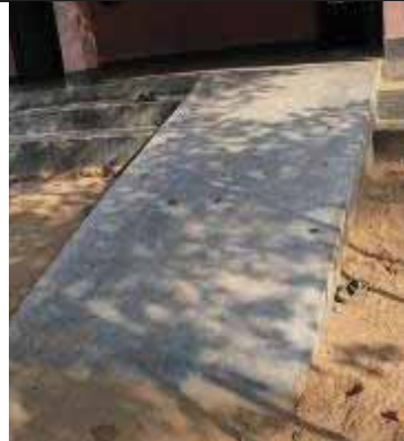
Ramps for disabled not made available in all schools or if present are broken
