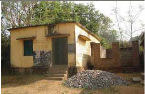
Kitchen being constructed between classrooms—a potentially hazardous situation (Mitu Kereda PS, Rayagada district)
