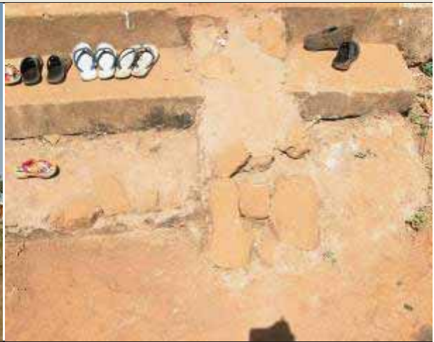
Status of ramps: Non-existent or broken
