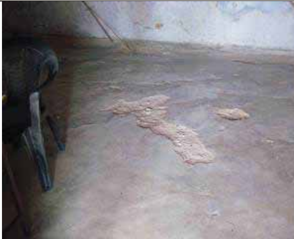
Chipped floor of classrooms
