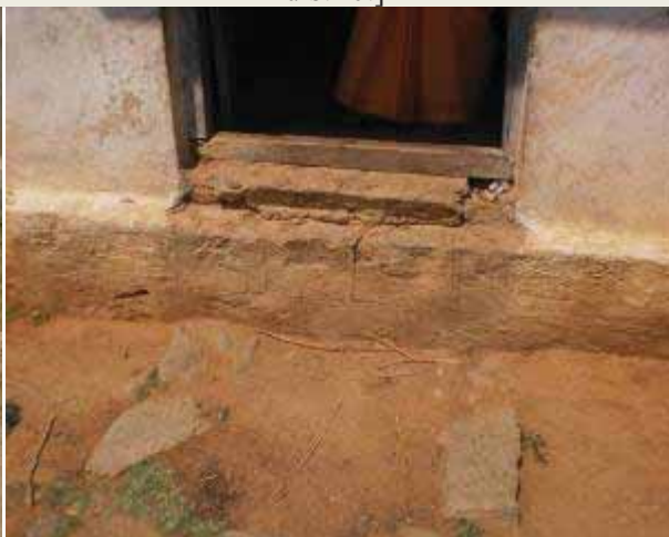
Unsafe access into classroom in a Primary School. Broken and rundown infrastructure a common sight
