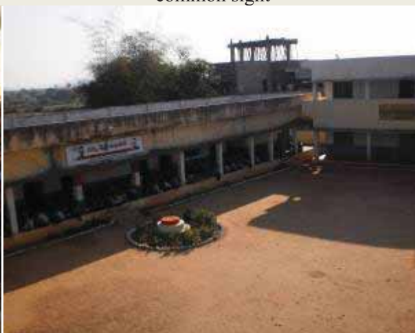
The roof of the residential school is used by the girls to dry their clothes and has no parapet walls on its sides [Jangamreddypally TWAHS(G), Mahabubnagar district]
