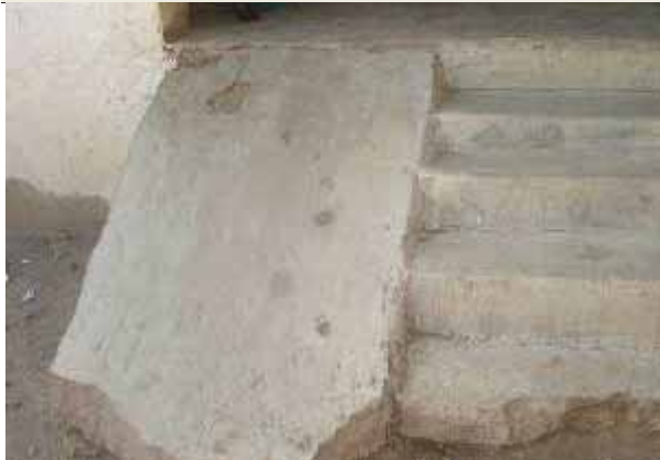
Ramps are either non-existent or were found to be broken in most schools
