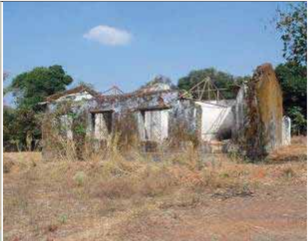
Dilapidated school building of Kenduguda TWPS, Visakhapatnam district
