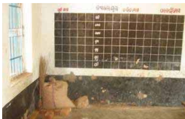
Classrooms dilapidated and used as storerooms
