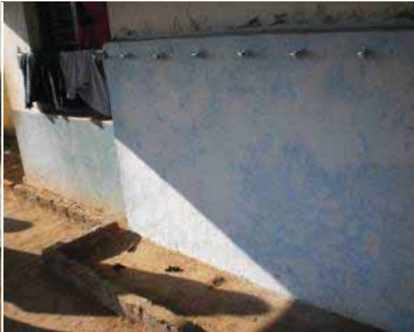
Lack of hygiene is a serious issue in residential schools. The area where taps for drinking water have been provided were dirtied by dogs [Jangamreddypally TWAHS(G), Mahabubnagar district]
