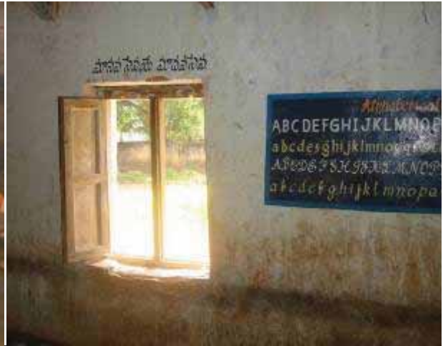
Broken windows and poor infrastructure a common sight
