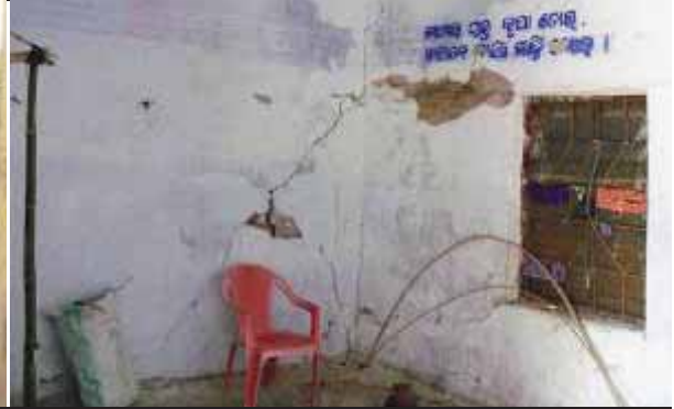
Cracking roof and walls a safety hazard to children
