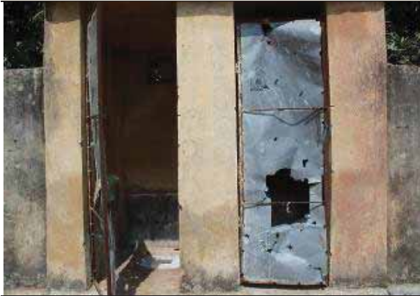
Toilets broken down, lack water and are mostly non-functional
