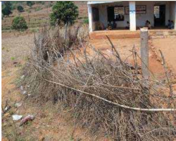
A boundary wall for a Primary School made of sticks and twigs. In several schools boundary walls were absent
