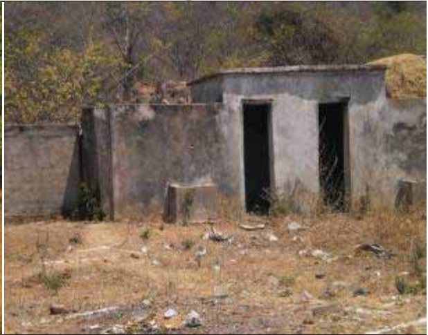
Disused or semi-constructed toilets
