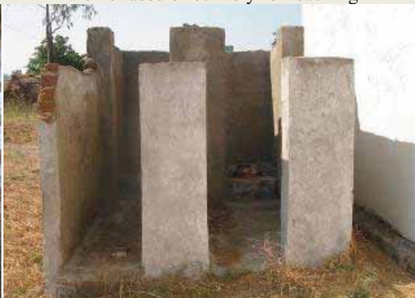
Semi-constructed and non-functional toilets were a common sight in all districts visited
